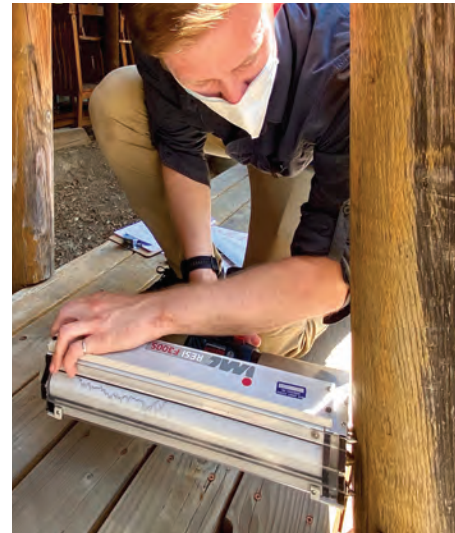
Engineer conducts wood density test to measure possible deterioration in balcony post.
