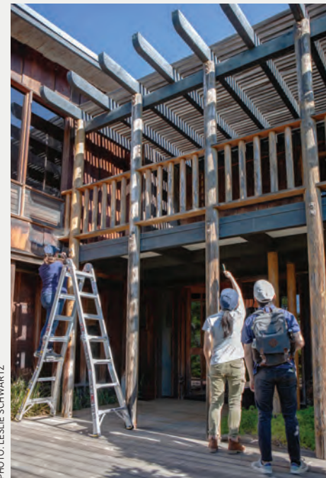
South-facing balcony is severely deteriorated and has been restricted for occupants, per WJE's recommendations.
