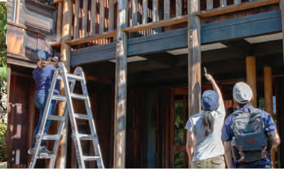
Malooof Roof Repair and Reconstruction plans have been approved by National Park Service and California's State Historic Preservation Officer. Onsite work, including balcony restoration, is slated to begin in spring 2024.
