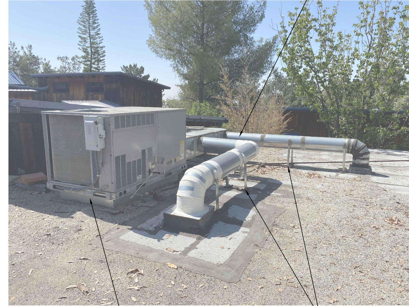
2 Rooftop Equipment and Duct at Workshop 1 (West) Not to Scale
