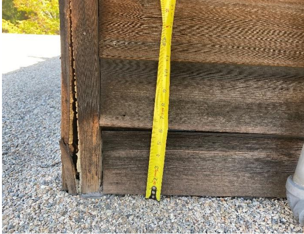
Figure 10. Horizontal siding with very little clearance at the Visitor Center/Gift Shop
