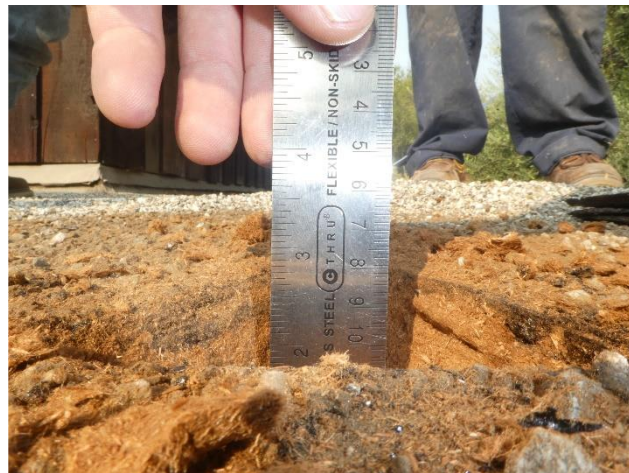
Figure 5. The depth of the roof core location, including the roof assembly and substrate measured approximately 2-3/4 inches.
