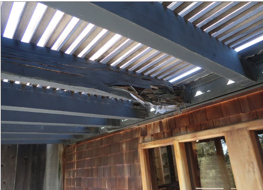
Image 18: Detail of deteriorating rafter at south balcony, view northwest (Chattel, 2022)
