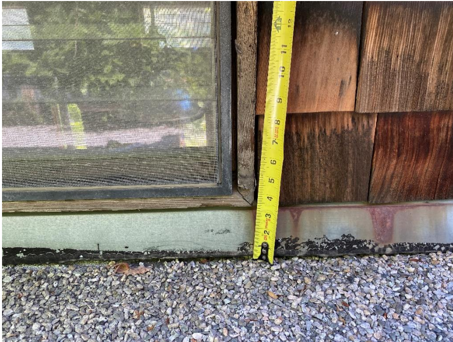
Figure 25. Example of very little available flashing height below existing window and shingle cladding.
