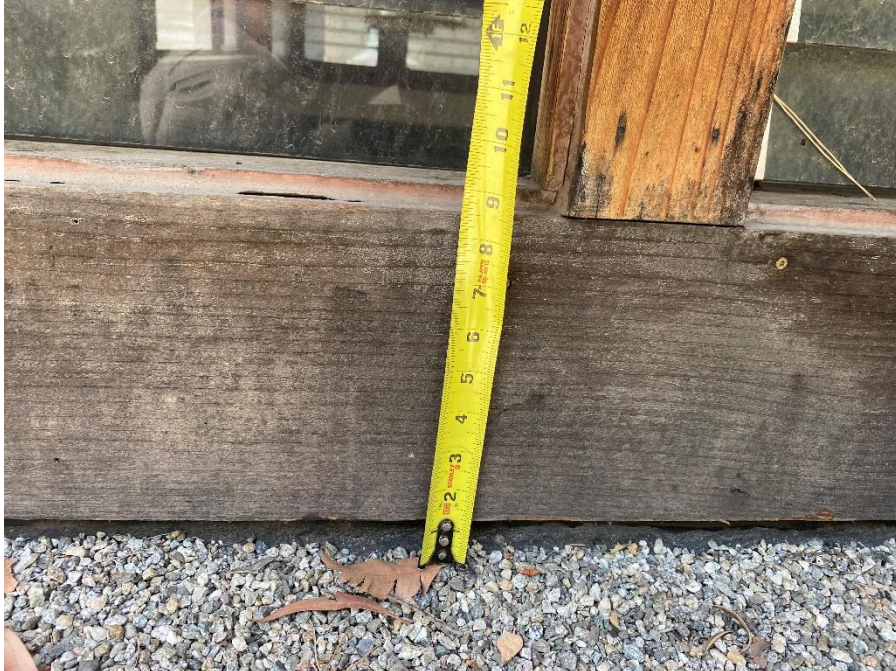
Figure 24. Example of very little available flashing height below clerstory window.
