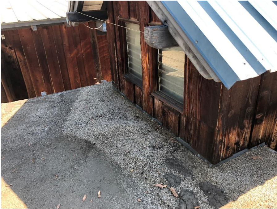
Figure 19. Example at rising wall with vertical siding and limited vertical flashing height below industry standard recommendations. This area is largely unseen from elsewhere on site.
