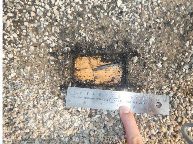
Figure 3. In most areas the roofing assembly was installed directly onto the wood roofing substrate, photograph from the Visitor Center.
