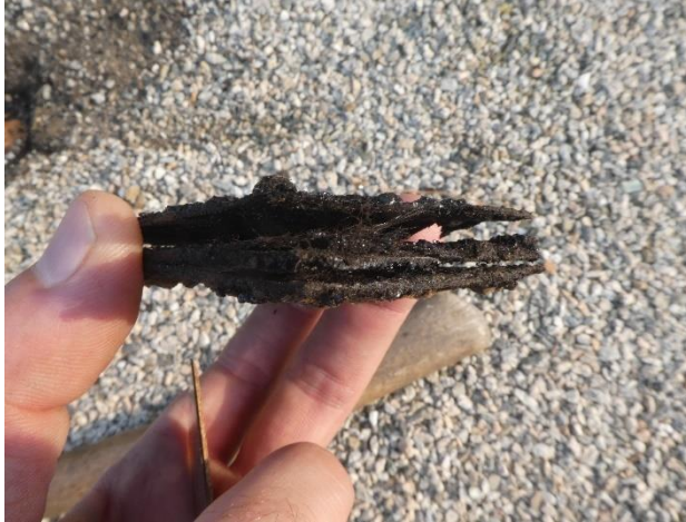
Figure 2. Three plies of the roofing felt were identified to be saturated and partially separated with hot-applied asphalt waterproofing
