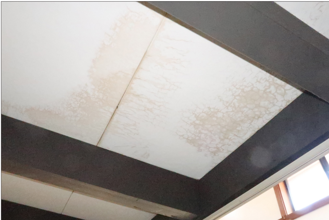
Image 26: Detail of water damage at ceiling (Chattel, 2022)
