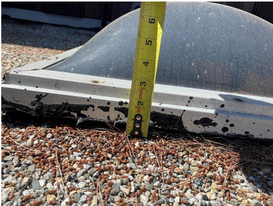
Figure 26. Example of very little available flashing height at skylight.
