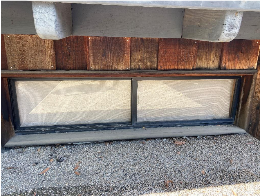
Figure 23. Example of very little available flashing height below existing window.
