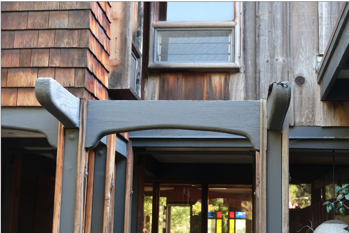
Image 16: Detail of rafters at Main House north elevation entrance, view south (Chattel, 2022)
