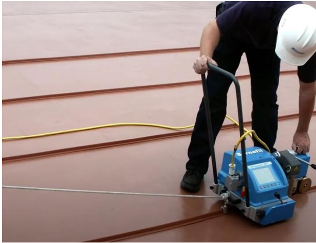
Figure 16. PVC roof membrane with Décor strips added to simulate standing seam metal roof
