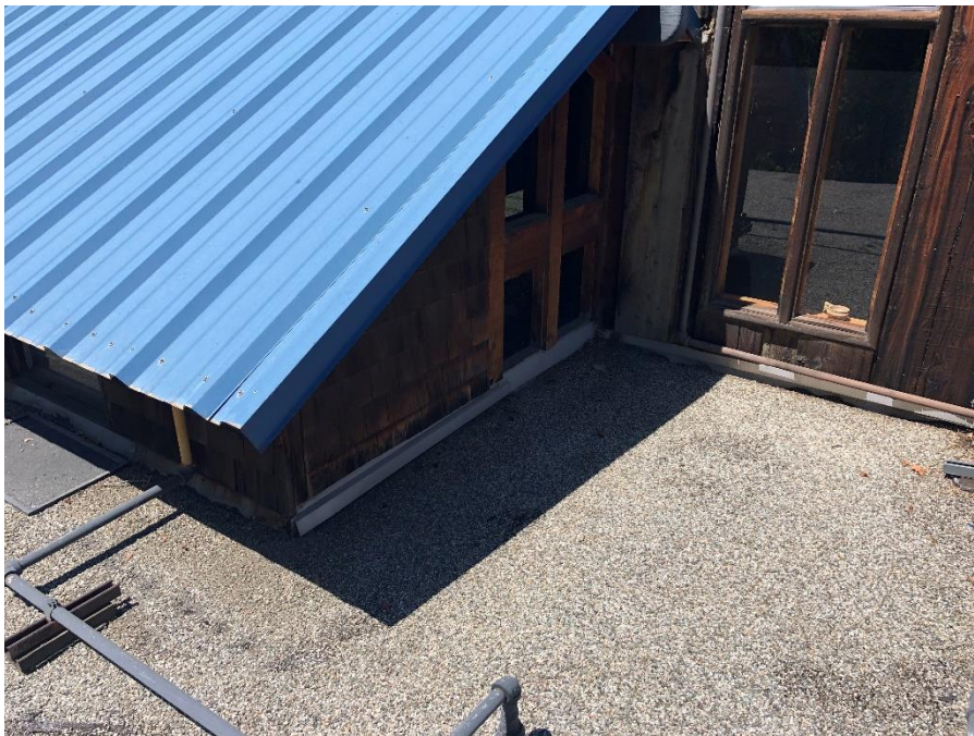
Figure 22. Example at rising wall with window and shingle cladding along with limited vertical flashing height below industry standard recommendations.
