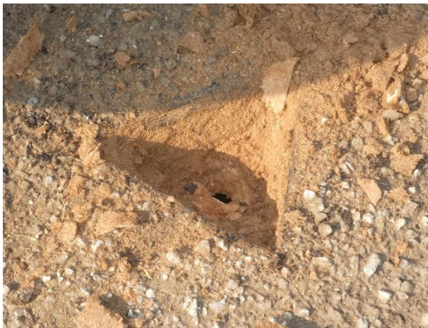
Figure 4. Roof core created at the conference room, north. The roofing assembly was installed directly onto the insulation/fiberboard substrate. The roofing assembly was measured at approximately 1/2 inch.
