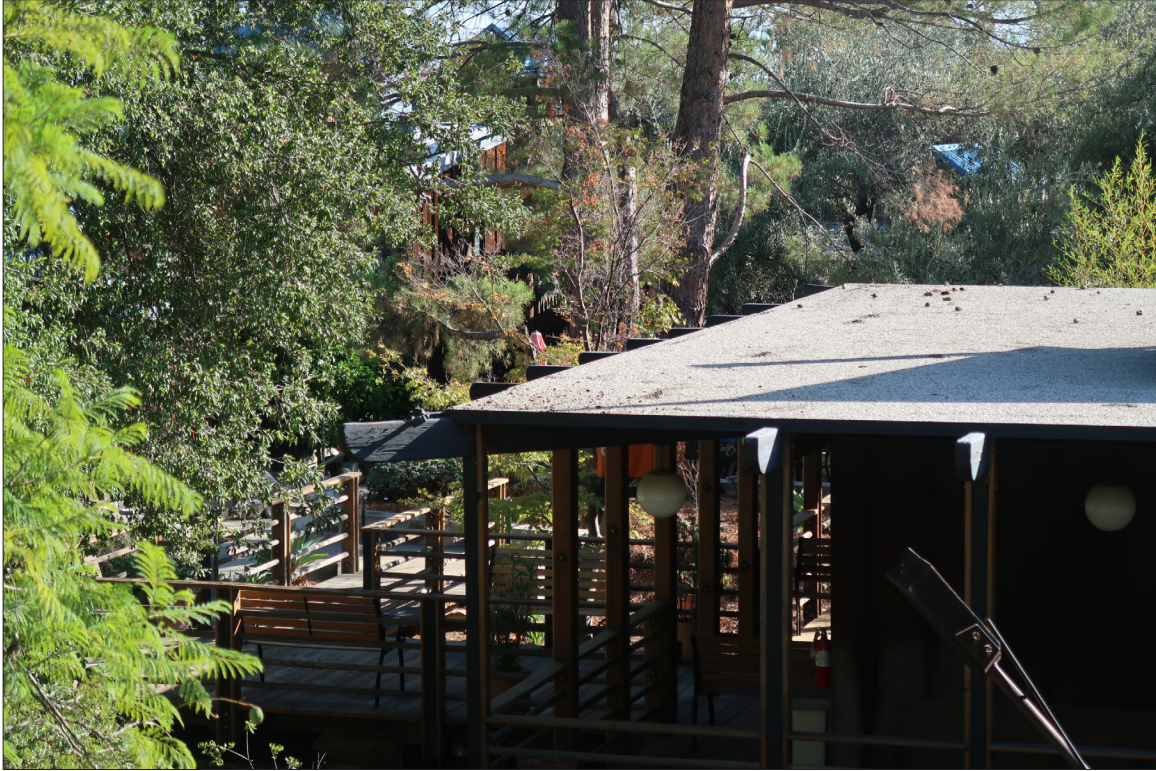
Image 29: Detail of built-up asphalt roof with gravel surfacing at Guest House, view southwest (Chattel, 2022)
