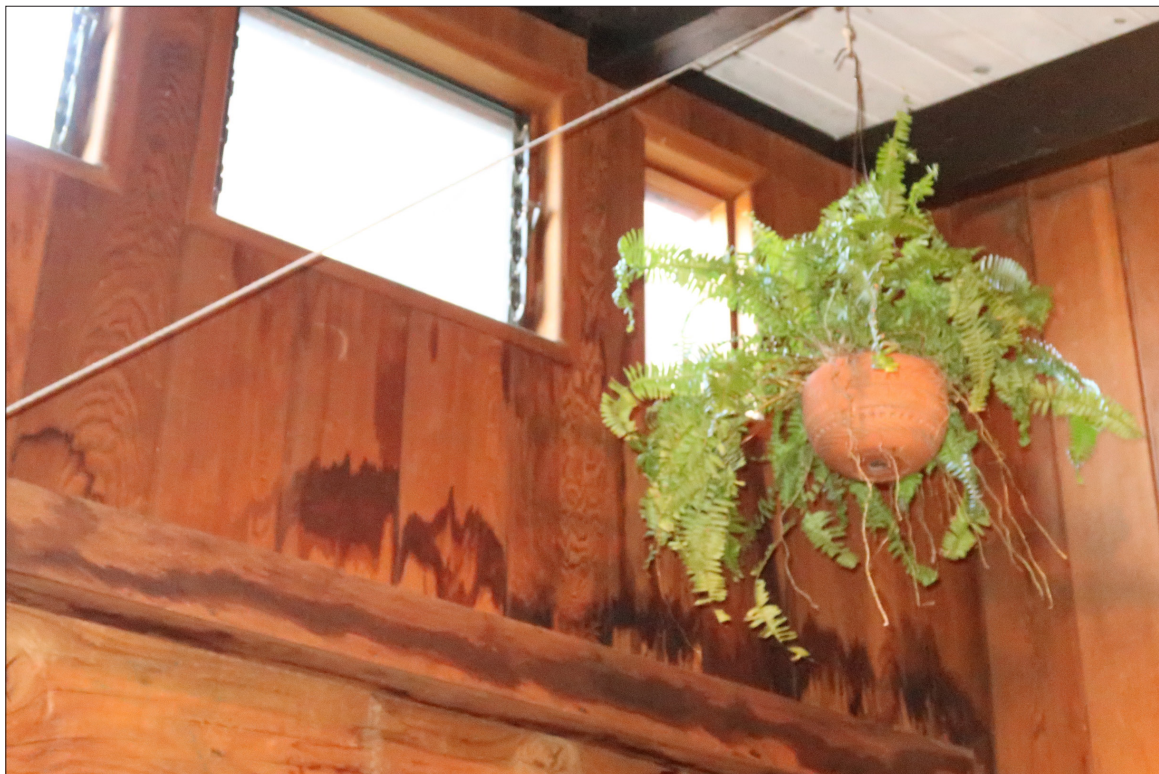
Image 24: Detail of water damage on wood clad walls (Chattel, 2022)
