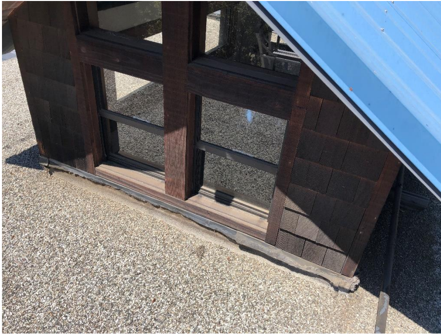
Figure 21. Example at rising wall with window and shingle cladding along with limited vertical flashing height below industry standard recommendations.
