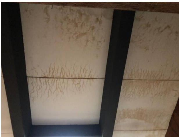
Figure 6. Water damaged fiberboards near the kitchen skylights
