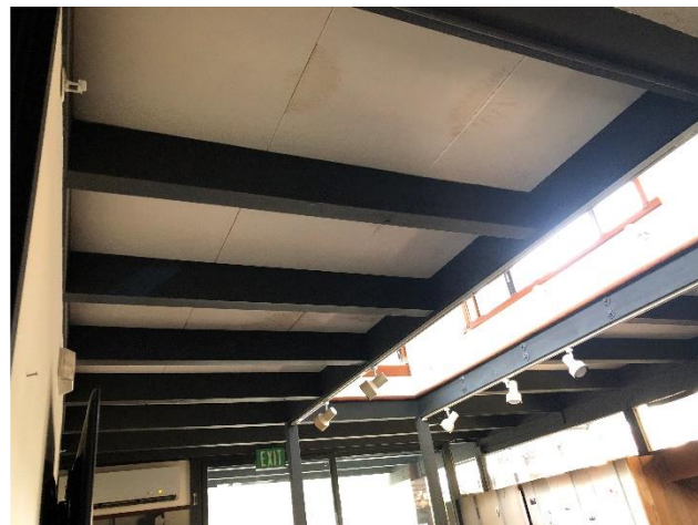
Figure 7. Water damaged fiberboards in the conference room
